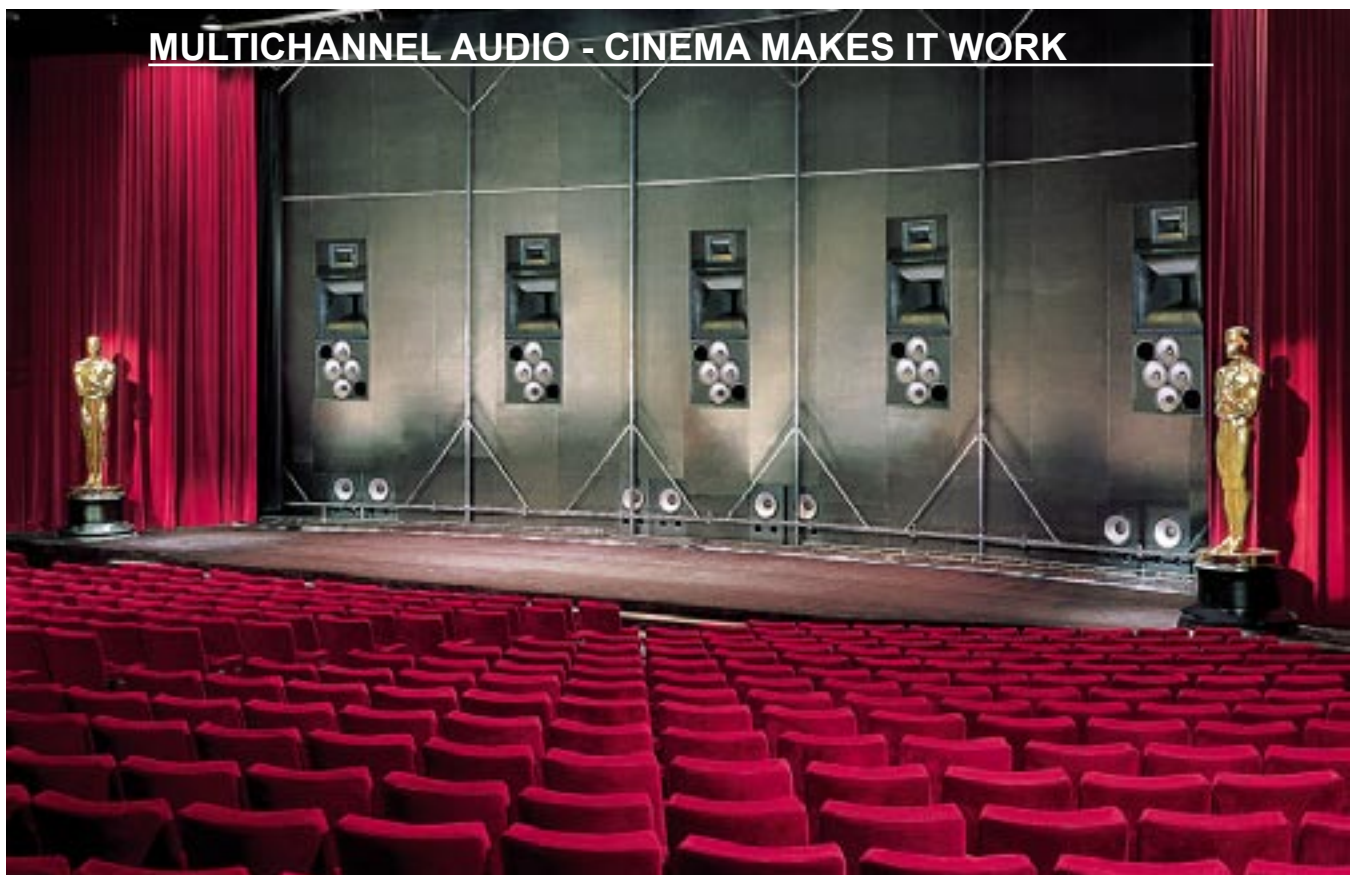
Figure 3. The Academy of Motion Picture Arts and Sciences, Samuel Goldwyn Theater, showing five front channels of JBL loudspeakers and eight 18-inch subwoofers for low-frequency effects (LFE). All of this, of course, is hidden behind a perforated screen. Twenty-four surround loudspeakers complete the installation.
